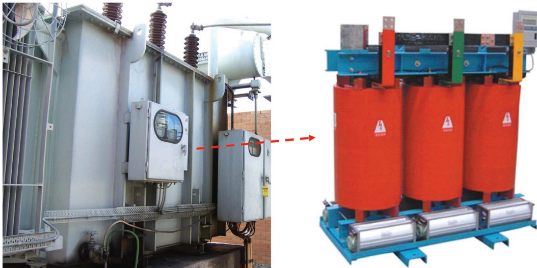
Fig. 16. Power transformer (exterior view and interior windings).
