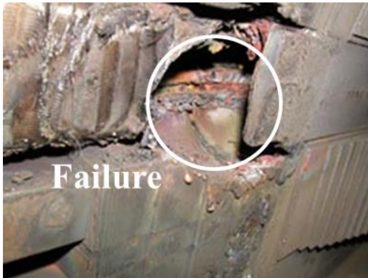
Figure 3-3. Failure of a power generator stator
